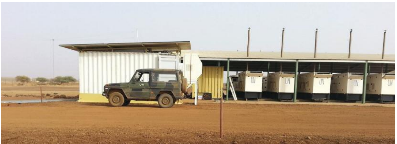
ESTechnologies Smart Energy plant in Mali supplying the Netherlands Camp
